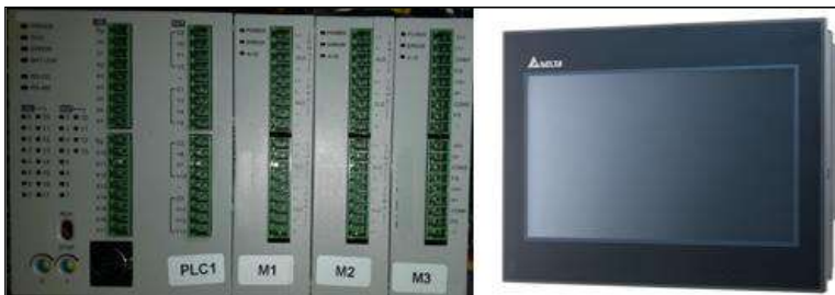
Figure 2: Plc, Plc Modules and Human Machine Interface.
