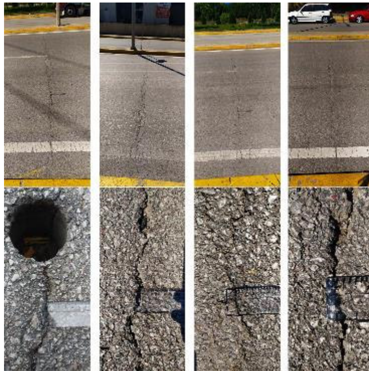
Figure 8. In situ examination of reflection cracks (2022)
