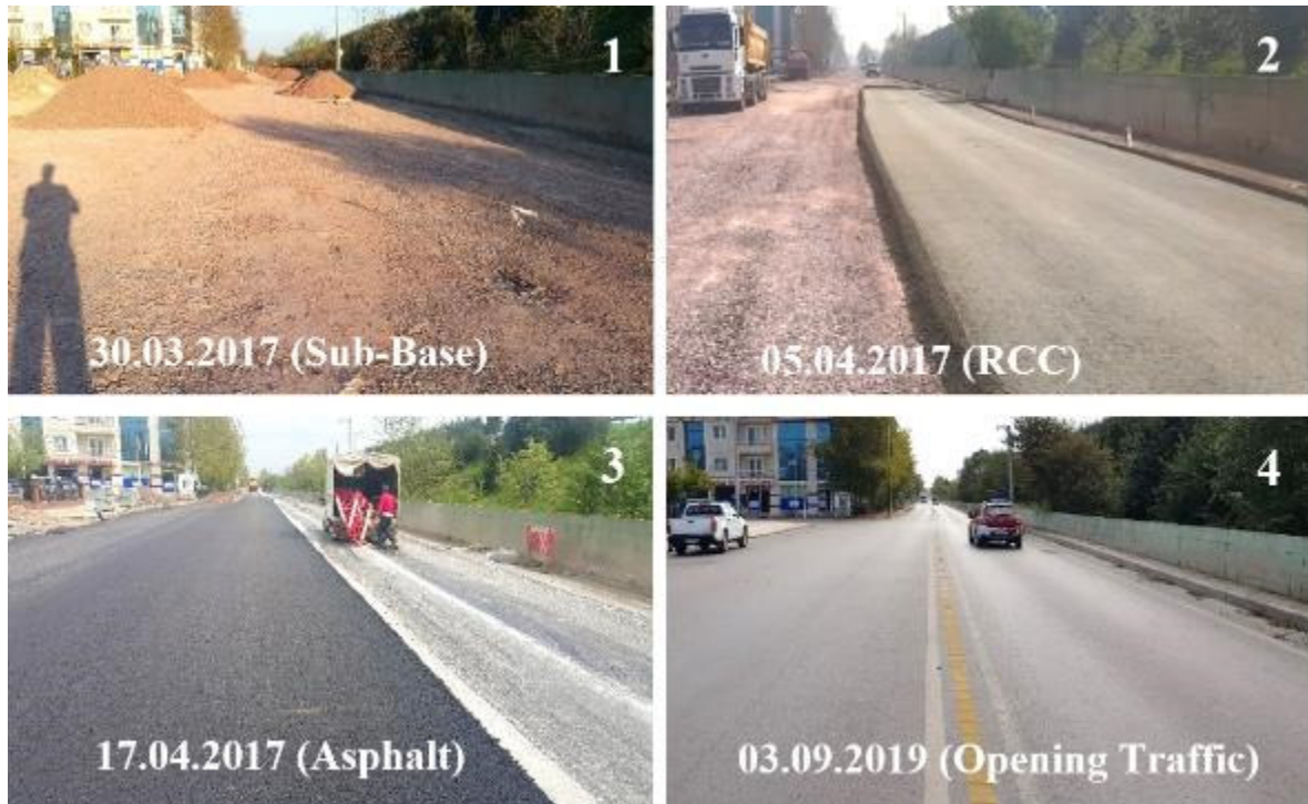
Figure 5. Construction of the pavement layers and the current state of the road
